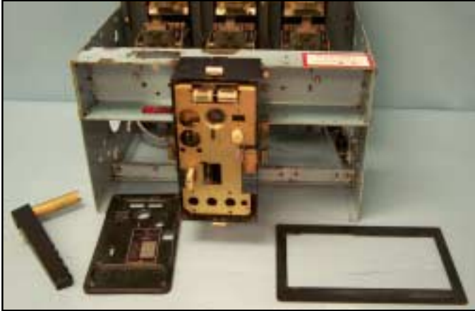
Fig. 3 Charging Handle, Face Plate, and Floating Trim Removed from the Breaker.
