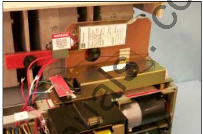
Fig. 54 Aux. CT Module Assembly Installed on the Breaker and Preliminary Routing of the Sensor Harness, DTA Wires, and CPT Wires.
