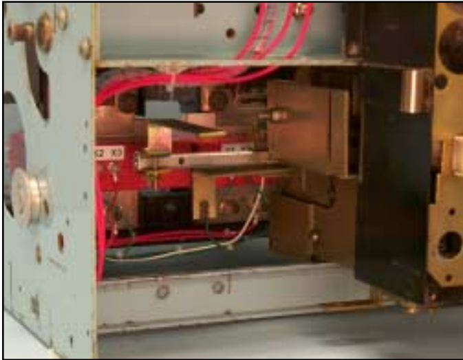
Fig. 34 Overview: Trip Finger Installed in the Breaker - Long Trip Shaft.
