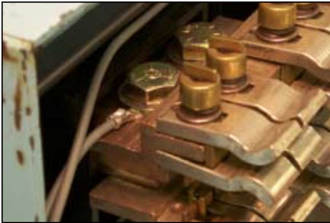
Fig. 31 HV Wires Connected to Top Secured Finger Clusters.
