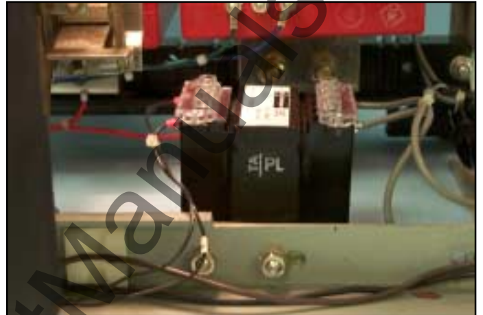
Fig. 18 Overview: Breaker Mounted CPT Installed in the Breaker.
