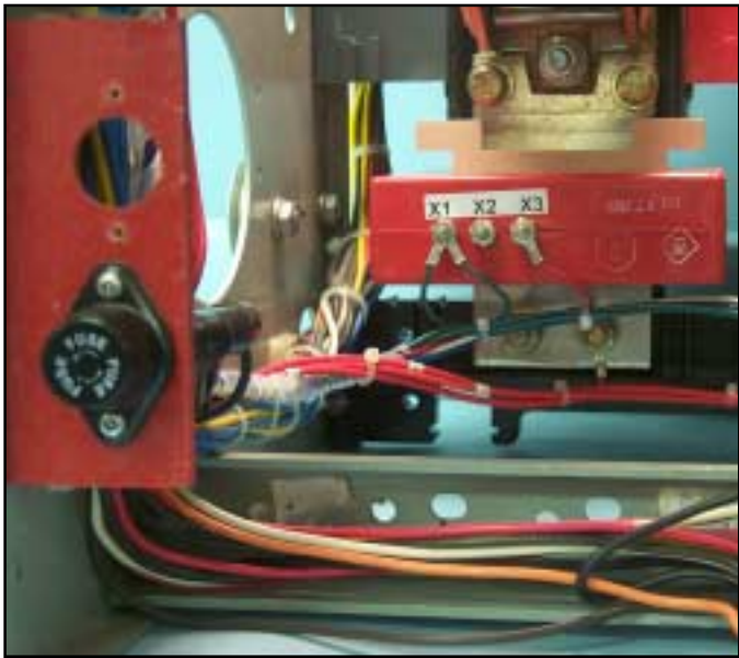
Fig. 17 PT Wires Secured to the Sensor Harness.
