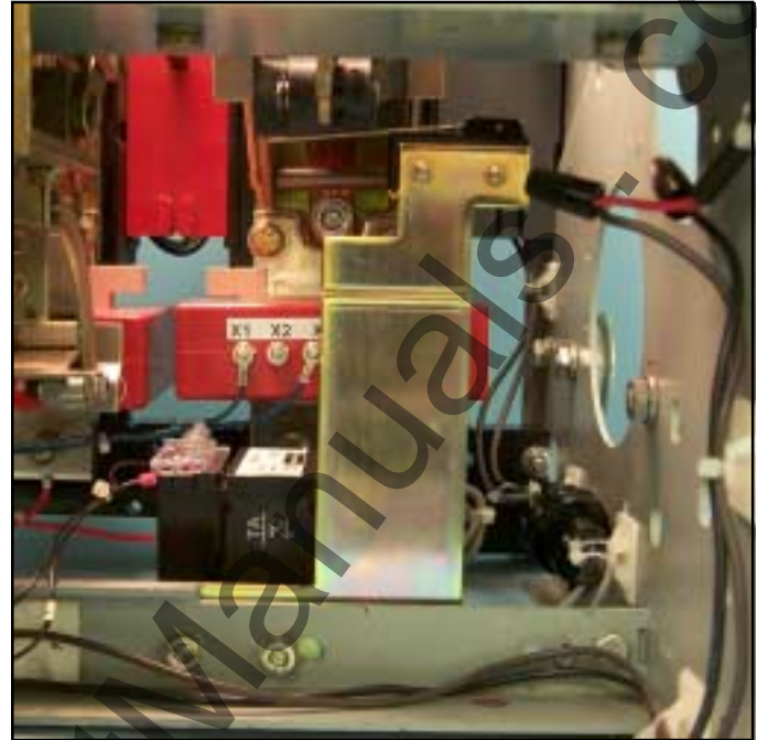
Fig. 27 Auxiliary Switch and CPT Assemblies Installed in the Breaker.
