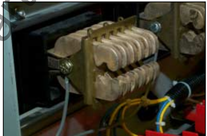
Fig. 30 HV Wires Connected to Side Secured Finger Clusters.
