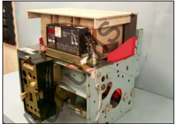
Fig. 59 Overview: External Harness Installed on the Breaker.
