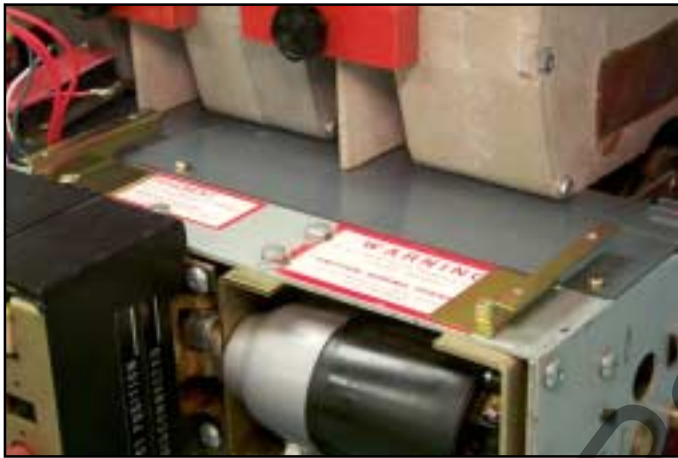
Fig. 53 Aux. CT Module Mounting Brackets Installed on the Breaker.
