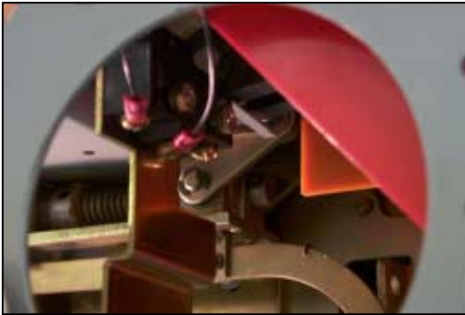
Fig. 61 External Harness Wires Connected to the Auxiliary Switch.
