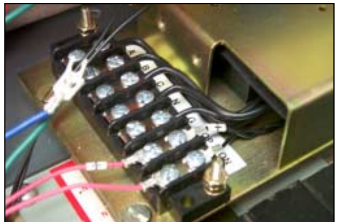
Fig. 55 DTA Wires Connected to the Aux. CT Module Terminal Block.
