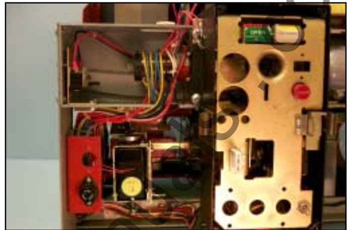
Fig. 49 Routing and Securing of the Original and New Wiring.
