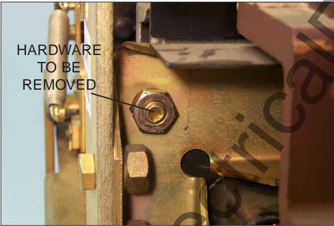
Fig. 10 Location of the Breaker Backplate Mounting Hardware.
