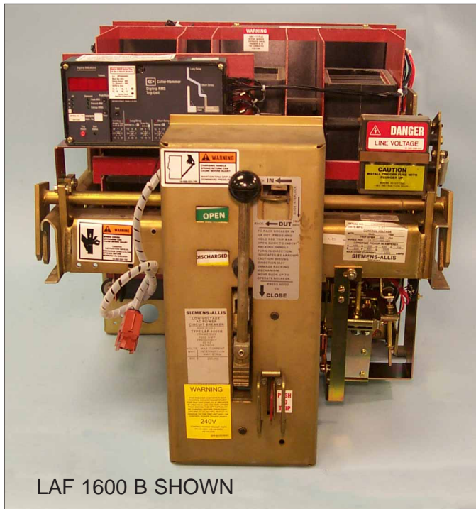
Fig. 76 Overview: Breaker Ready for Testing.
