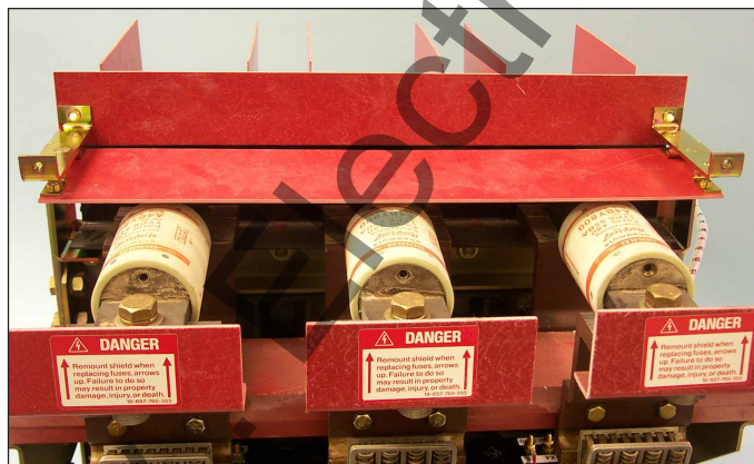
Fig. 14 Bottom Aux. CT Module Insulation Barrier Assembly Installed on the Aux. CT Module Mounting Brackets.
