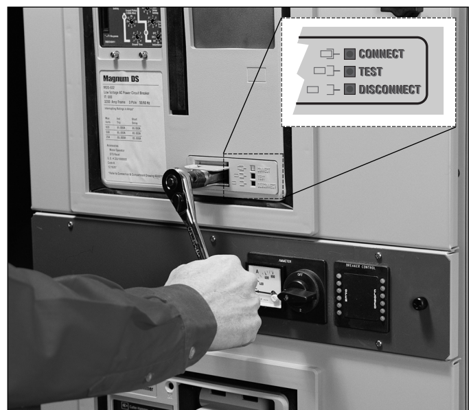
Figure 2-11 Circuit Breaker Being Levered
