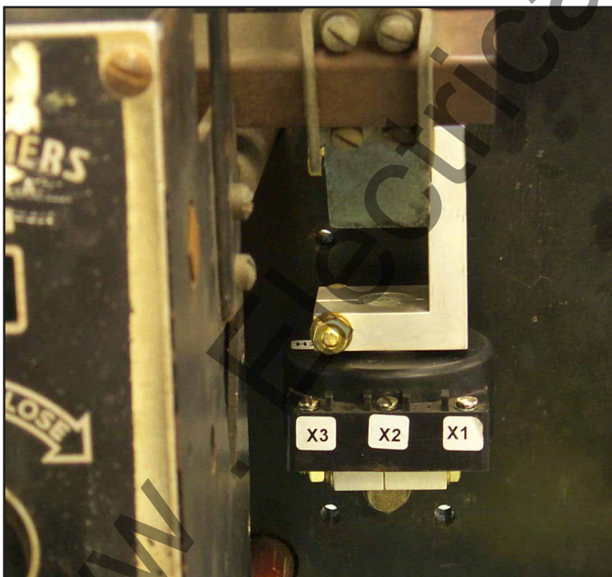
Fig. 12 Sensors Installed in the Breaker with Copper Adapter Cylinders In Place.
