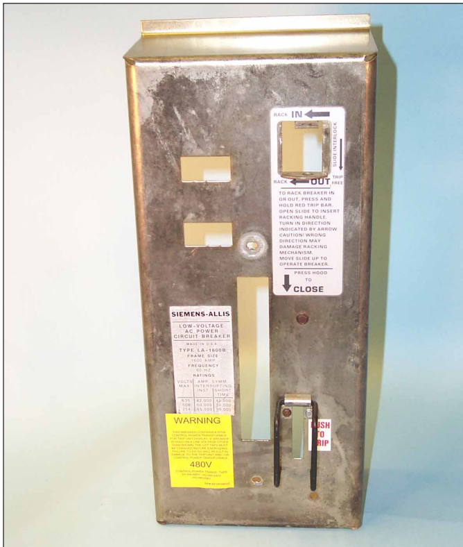
Fig. 45 CPT Voltage Label Installed on the Breaker Cover.
