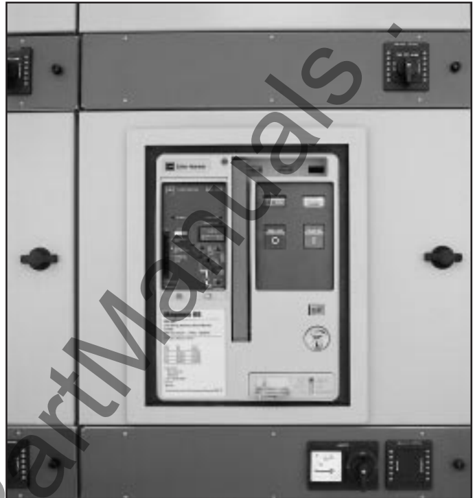
Figure 3-2 One High Magnum DS Breaker in Connected Position
