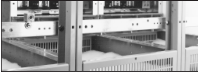
Figure 3-11 Ground Bus in Cable Compartment
