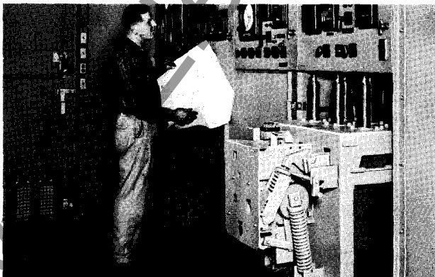
AISLE SPACE is large enough for two breakers to pass side by side.
