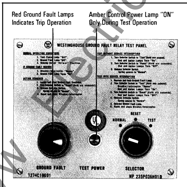
Fig. 4 Ground Fault Test Panel ①
