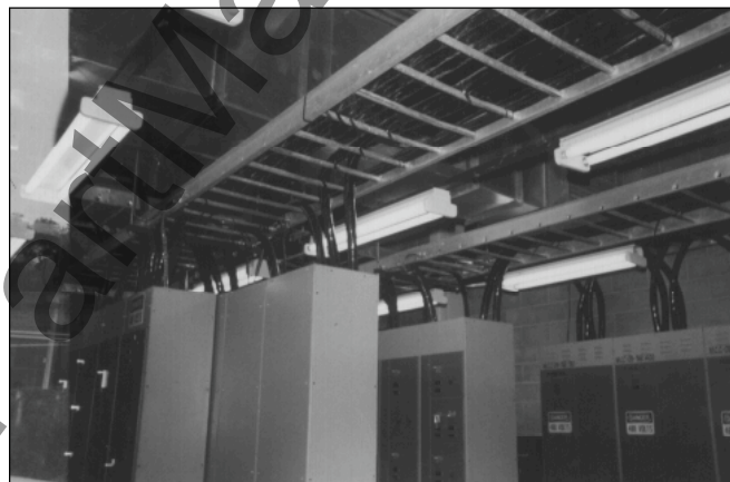
Cables Entering and Exiting Motor Control Centers from Cable Tray Systems.
