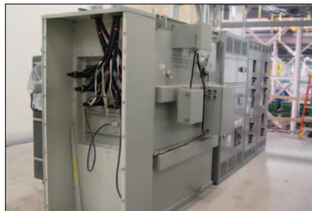
Indoor Power Center Transformer
