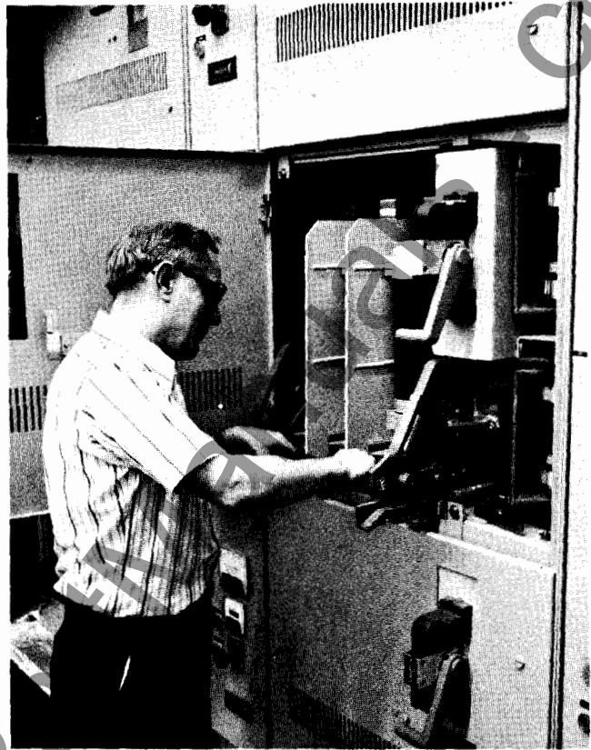
Fig. 45. Pulling on contactor positioning handle.
