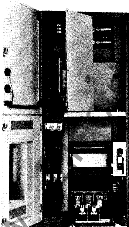
Fig. 67. Motor cable terminations in 42-inch-wide one-high enclosures.
