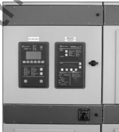
Devices Mounted on Instrument Compartment Door
