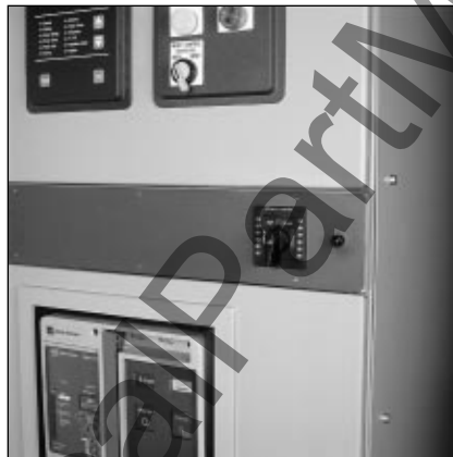
Devices Mounted on Secondary Terminal Compartment Door
