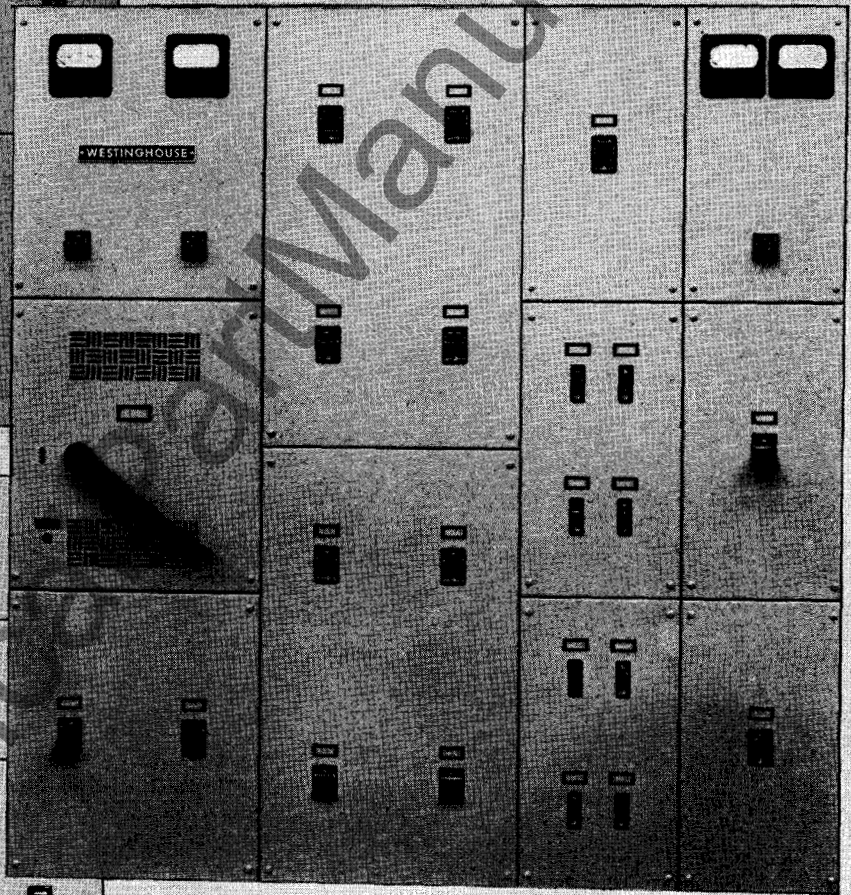
90 1/2 Inch High Switchboard using DA-50 and AB Types F, G, K and L Frames Manually Operated Circuit Breakers.
