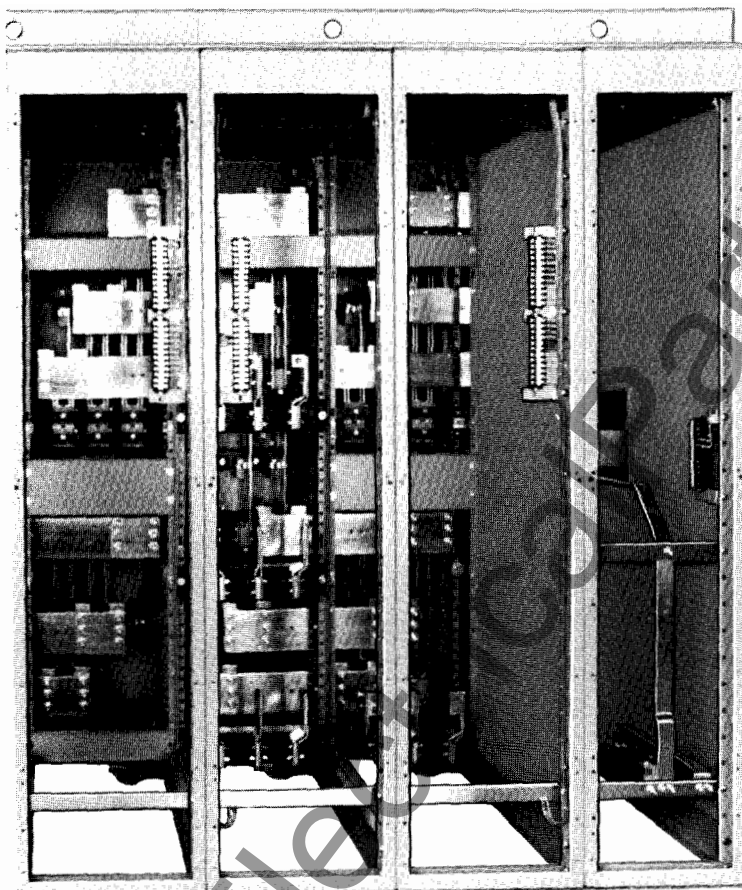
Bus and Cable Compartment with Barriers Removed
