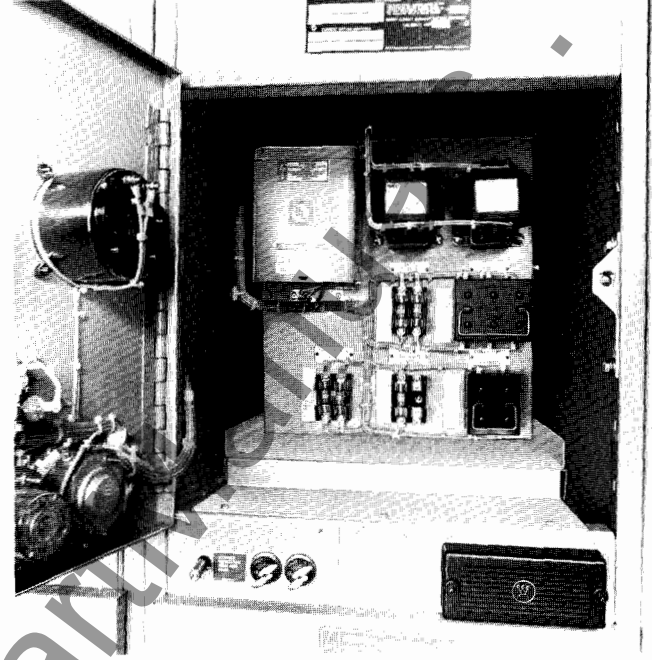
Potential Transformer and Control Power Transformer with Primary and Secondary Fuses
